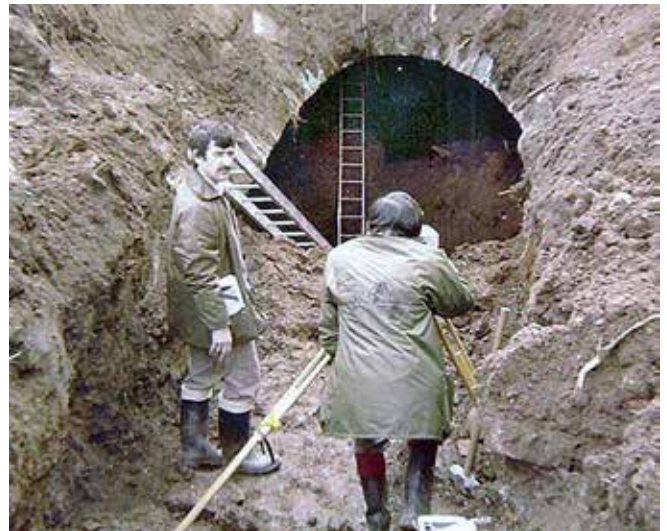
The northern end of Law Tunnel was excavated in 1981 for a survey prior to the adjacent housing being built.
